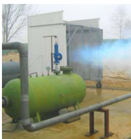
Safety valve test Bench
