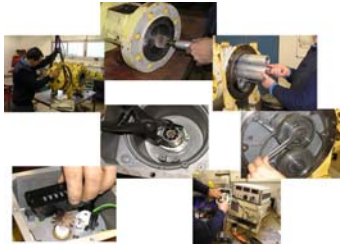
Meter repairing workshop
